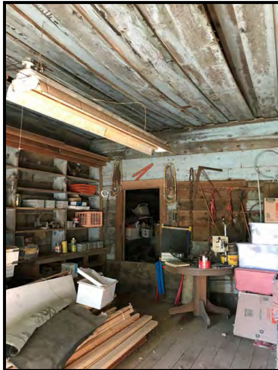
Photo 7. Interior view, Mountain House Historic District, Grocery Store/Post Office, looking northeast (Photo by Corri Jimenez).
